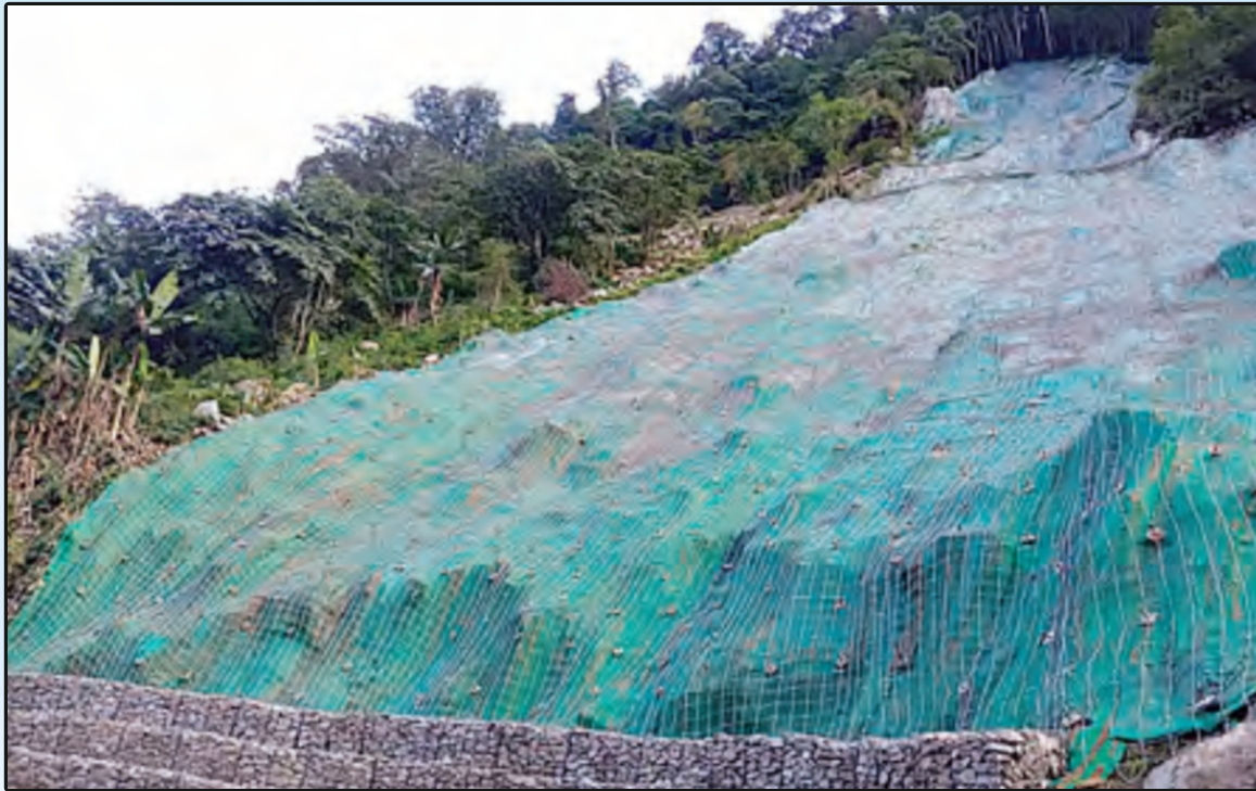
Biodegradable Coir Reinforced with Gabion Wall between Y Jn and Gelensiniak on Road TCC-Maza in Arunachal Pradesh
