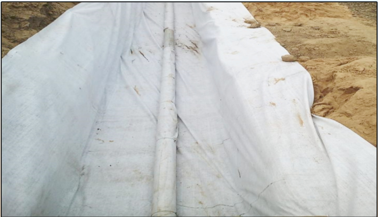
Sub-Surface Drainage System at Barrackpore Runway in West Bengal
