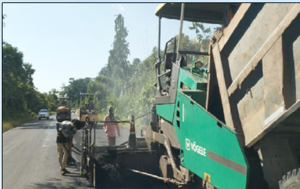
Laying of Bituminous Layer using Plastic Waste on Roing-Koronu-Paya Road in Arunachal Pradesh
