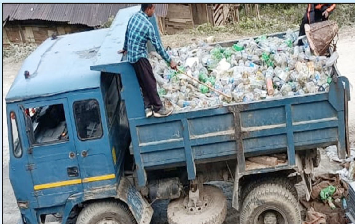
Collection of Plastic Waste for Resurfacing Works on Hapoli-Sarli-Huri Road in Arunachal Pradesh
