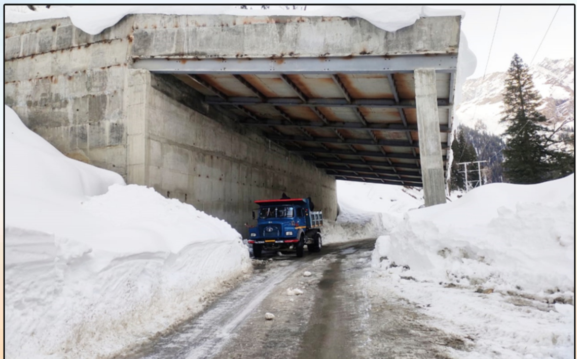
Snow Gallery at Km 9.13 on Approach Road to South Portal of Atal Tunnel in Himachal Pradesh
