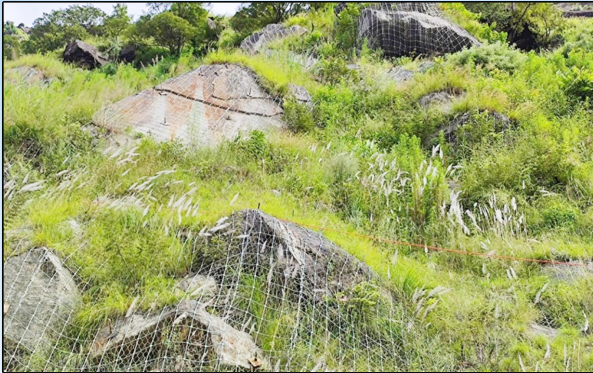
Secured Drapery on Joshimath-Mana Road in Uttarakhand
