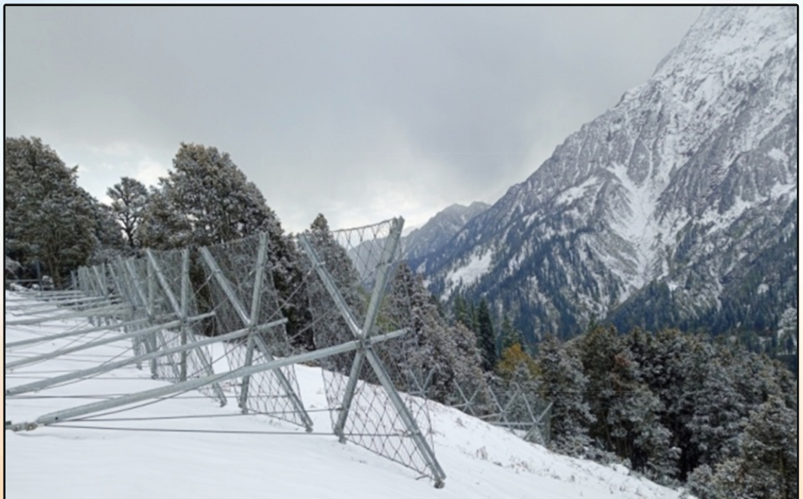
Snow Erodex System at Km 13.50 on Approach Road to South Portal of Atal Tunnel in Himachal Pradesh
