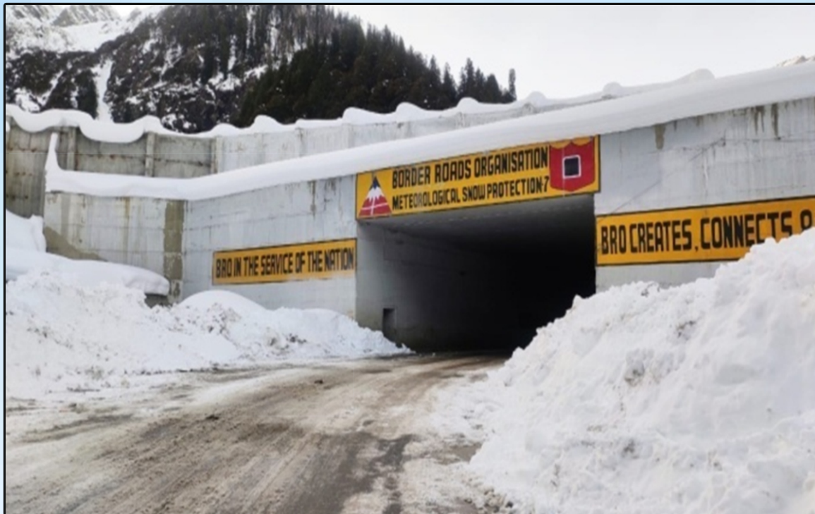
Snow Gallery at Km 8.77 on Approach Road to South Portal of Atal Tunnel in Himachal Pradesh
