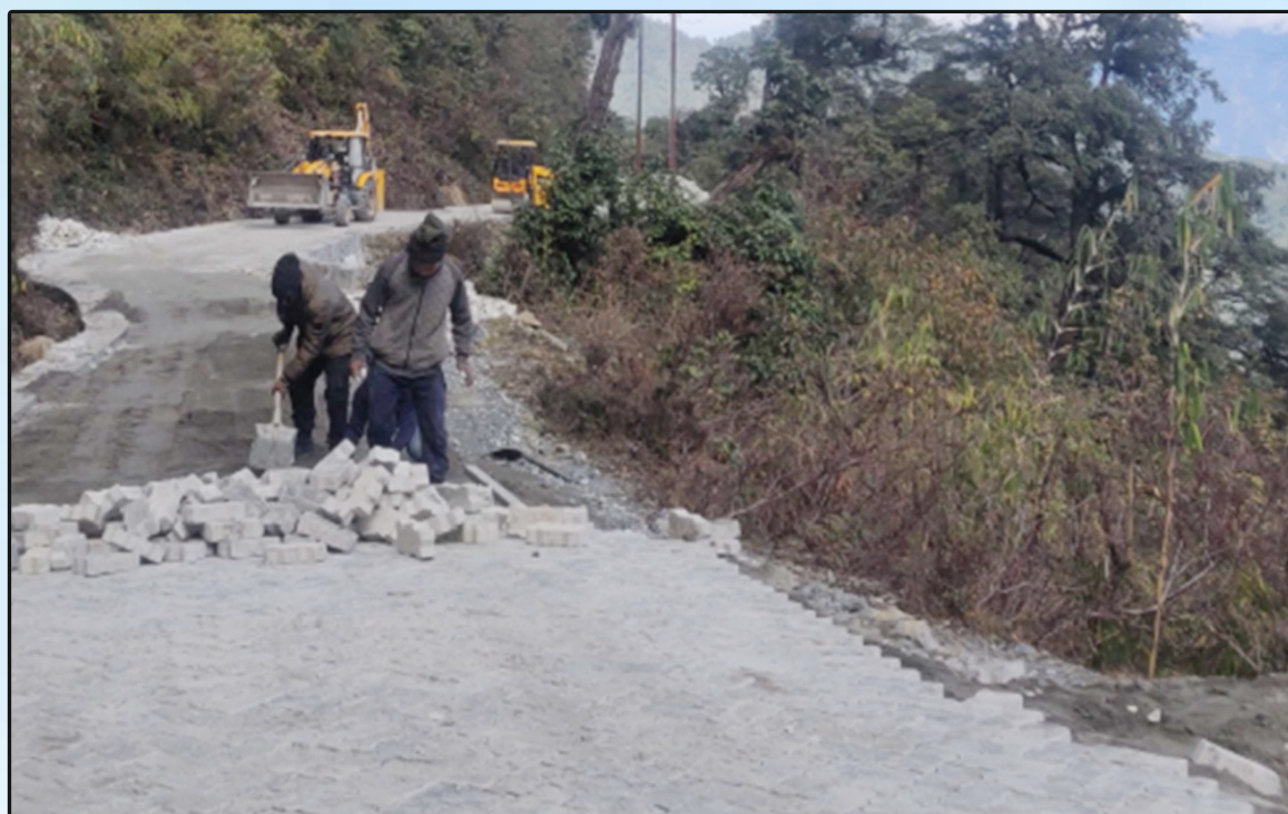
Laying of ILCB Pavement between Km 57 to 60 at Mayudiya Pass on Roing-Hunli Road in Arunachal Pradesh
