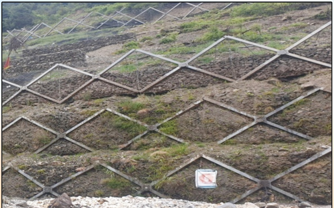
Use of Erdox-Cruciform Horizontal Consolidation Units on Kyachee GG-Nasar GG-Lungro GG (K-N-L) Road in Arunachal Pradesh
