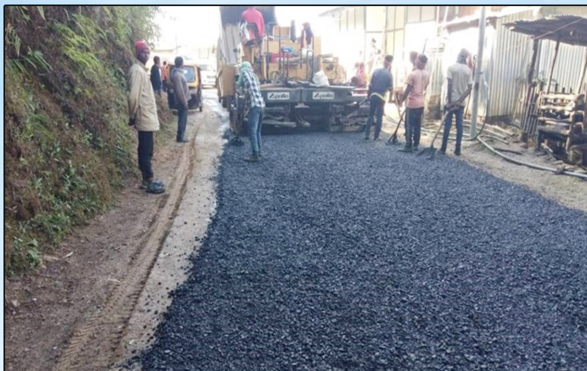
Laying of Bituminous Layer using Plastic Waste on Hnathial-Sangau-Saiha Road in Mizoram
