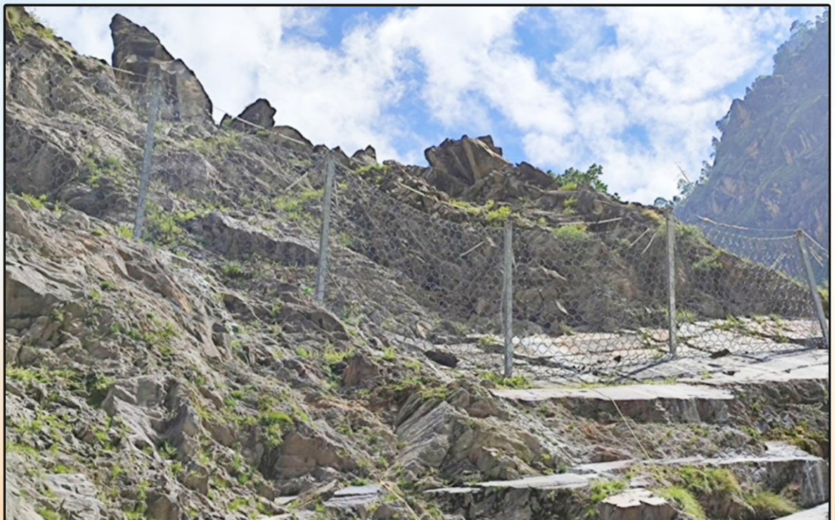
Dynamic Rockfall Barrier on Joshimath-Mana Road in Uttarakhand
