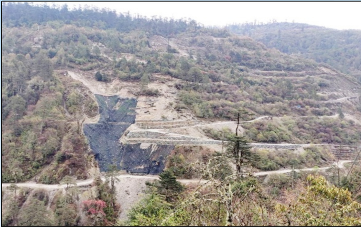
Use of Geotextile Material on Kyachee GG-Nasar GG-Lungro GG (K-N-L) Road in Arunachal Pradesh
