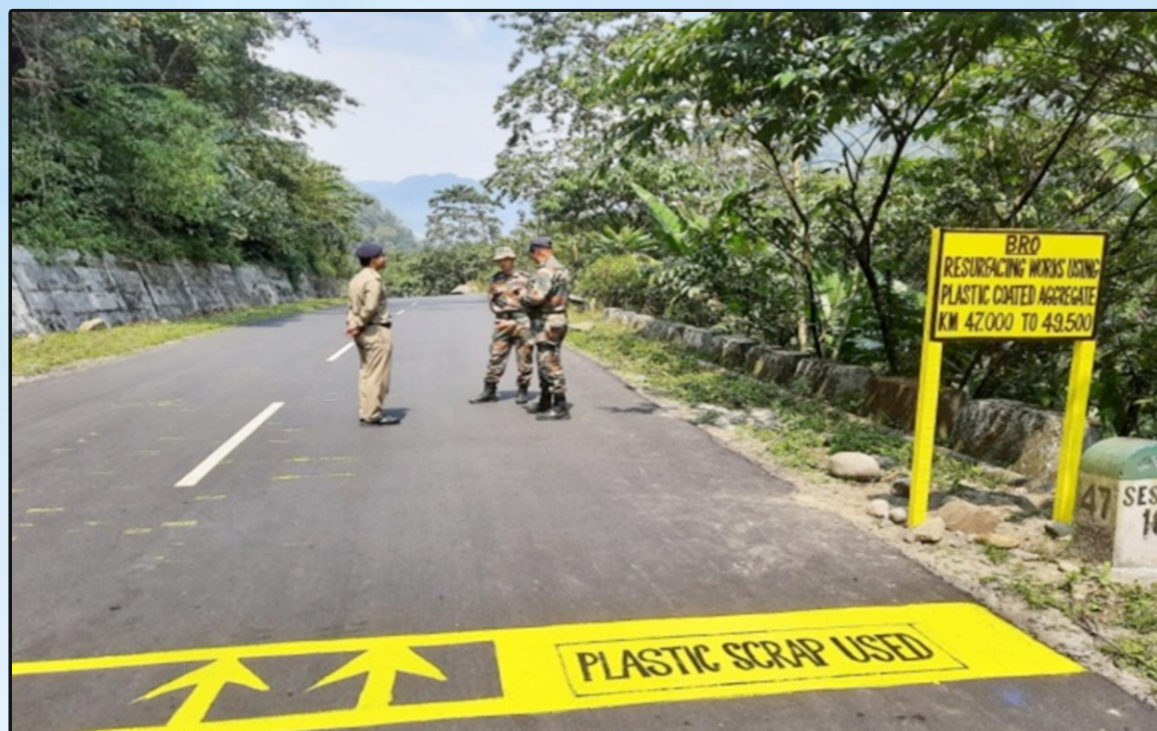
Completed Stretch using Plastic Coated Aggregates on Balipara-Charduar-Tawang Road in Arunachal Pradesh
