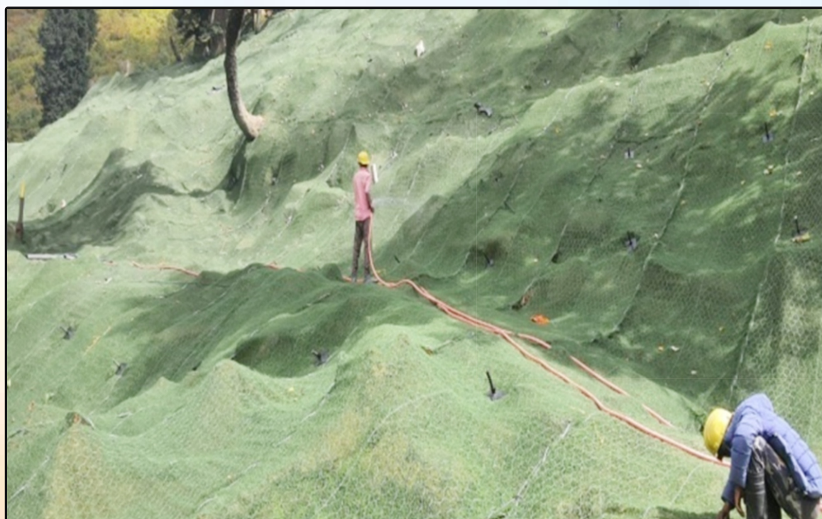
Reinforced Goemat on Approach Road to South Portal of Atal Tunnel in Himachal Pradesh
