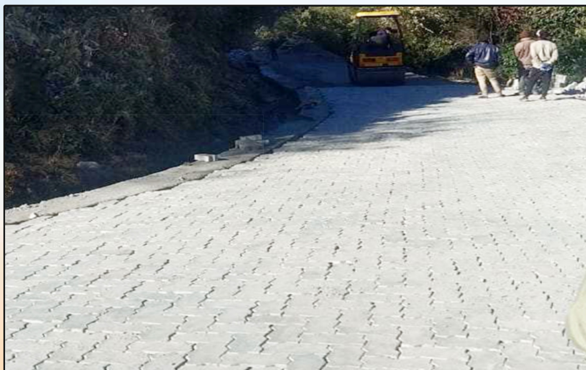
ILCB Pavement between Km 57 to 60 at Mayudiya Pass on Roing-Hunli Road in Arunachal Pradesh
