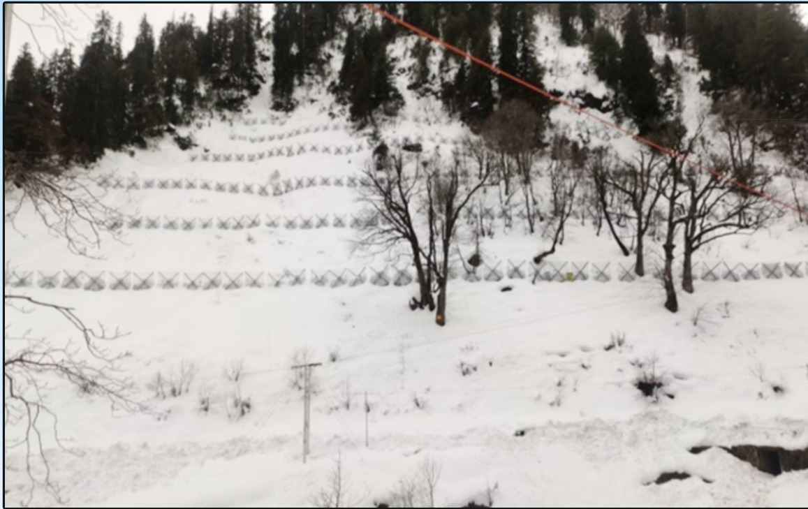
Snow Erodex System at Km 8.10 on Approach Road to South Portal of Atal Tunnel in Himachal Pradesh
