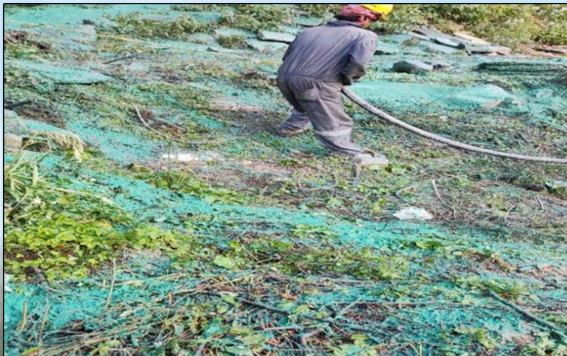
Hydro Seeding on Approach Road to South Portal of Atal Tunnel in Himachal Pradesh
