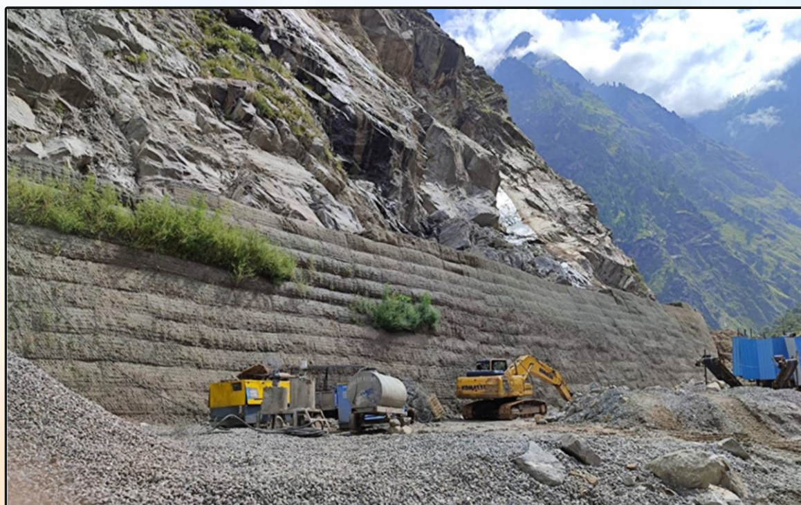
Rockfall Embankment on Joshimath-Mana Road in Uttarakhand
