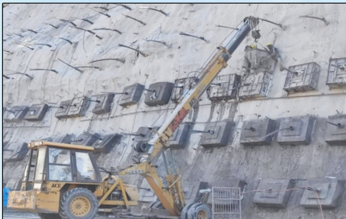
Pre-Stressed Cable Anchor on Approach Road to South Portal of Atal Tunnel in Himachal Pradesh
